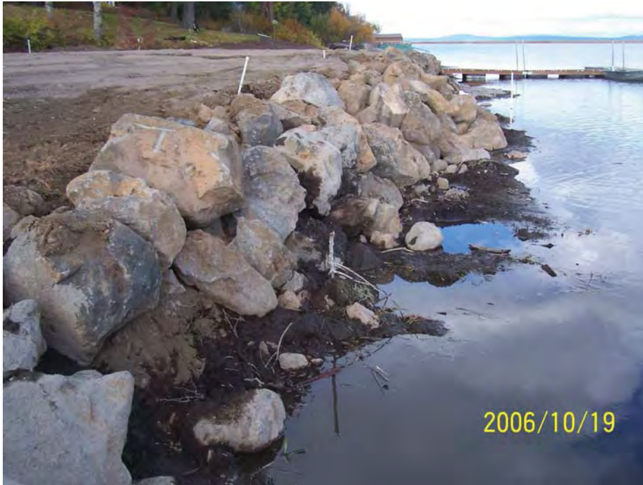
Figure 5. Fill violation in Upper Klamath Lake near Rocky Point on property T36S R6E, S2 tax lot 3000.
