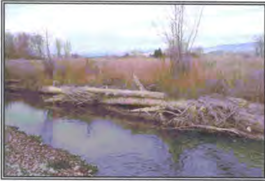
Figure 6.3: Bank stabilization/fish habitat structures are constructed with native materials including rootwads, deflector logs, and vegetation. Structures span from the scour depth to the bankfull elevation. Structure complexity benefits all age-classes of the target fish species. Young-of-year and juveniles use interstitial spaces while adults inhabit the deep scour pools that are formed around the rootwads.
