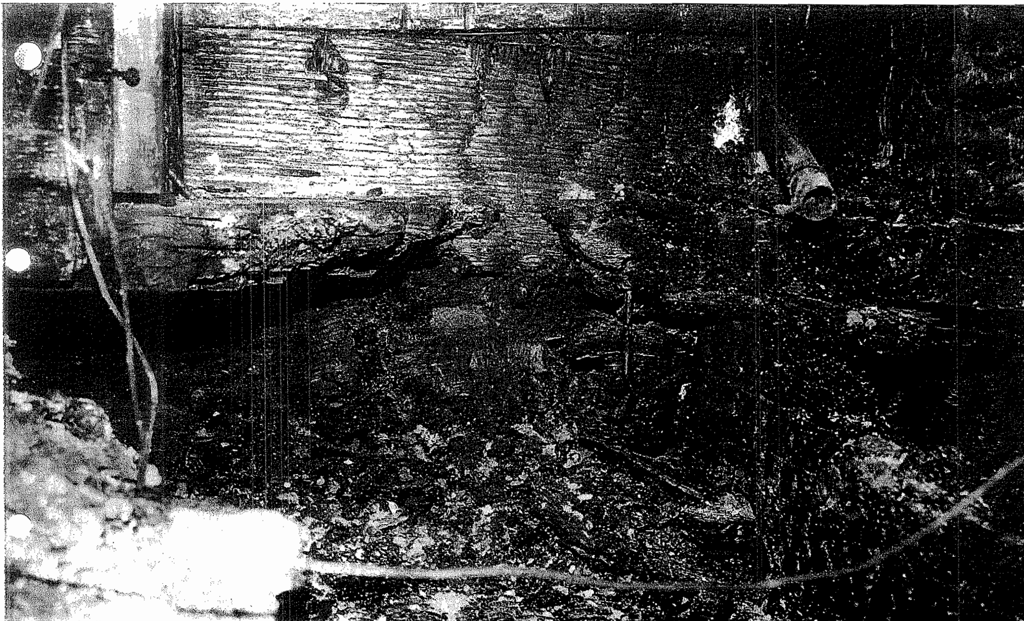
Photograph #75: The charring in the space between the two upright 2" x 4"s, shows the penetration down through the baseplate of the parapet wall. The original penetration was in proximity to the conduit shown in the upper right of the photograph. The arrow identifies the point of penetration through the baseplate that occurred during the propagation of the fire.
