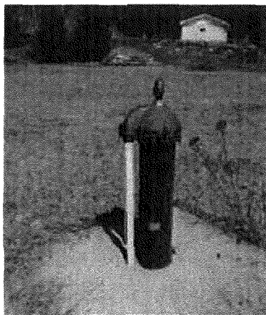
Well 2 (well field)
